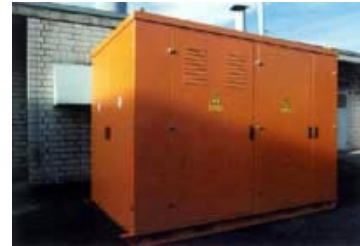
Kufen - Freiluft - Alu - Station 20 kV / 400 V / 50 Hz
